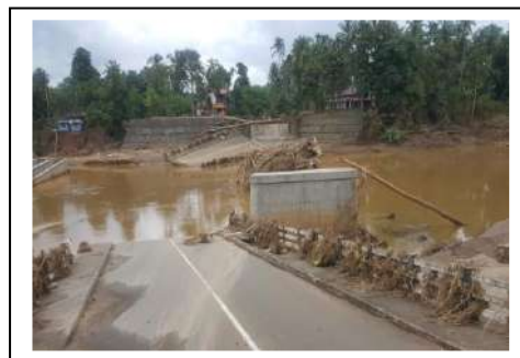
Fig 4 Collapsed Kaippini Bridge
