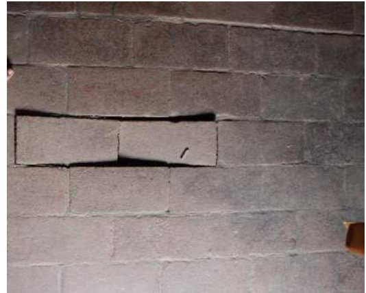
Tiles coming off
