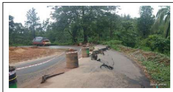
Fig 7 Damaged pavement in Mananthavady– Periya Road
