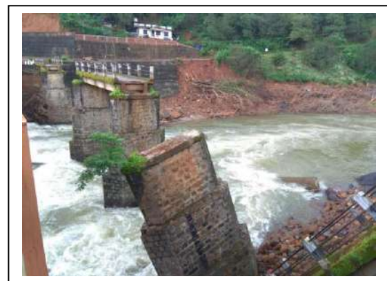
Fig 9 Collapsed Kacherikadavu old bridge
