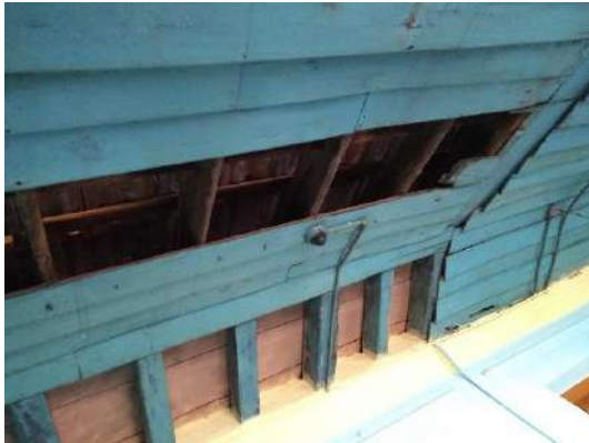
False ceiling coming off
