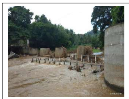
Fig 3 Collapsed Vannanthara Bridge
