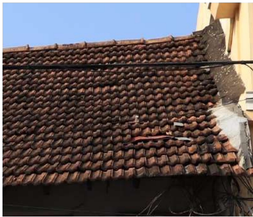
Broken tiles replaced by sheet
