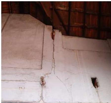
Crack on the wall
