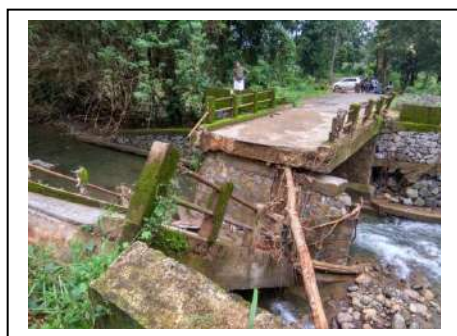
Fig 6 Collapsed Pothundi Bridge
